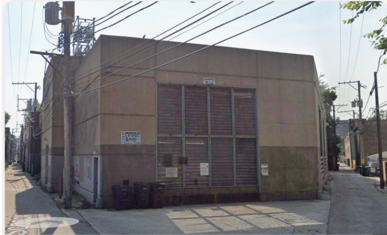
The current decommissioned substation infrastructure on site—serving as a stark physical reminder of the block's long-term utility footprint and the 2006 infrastructure failure.
